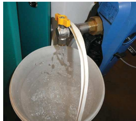
Rinsing using the rinsing tap
